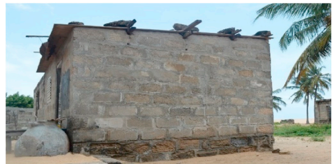
Fig. 10. Effect of erosion on buildings.
