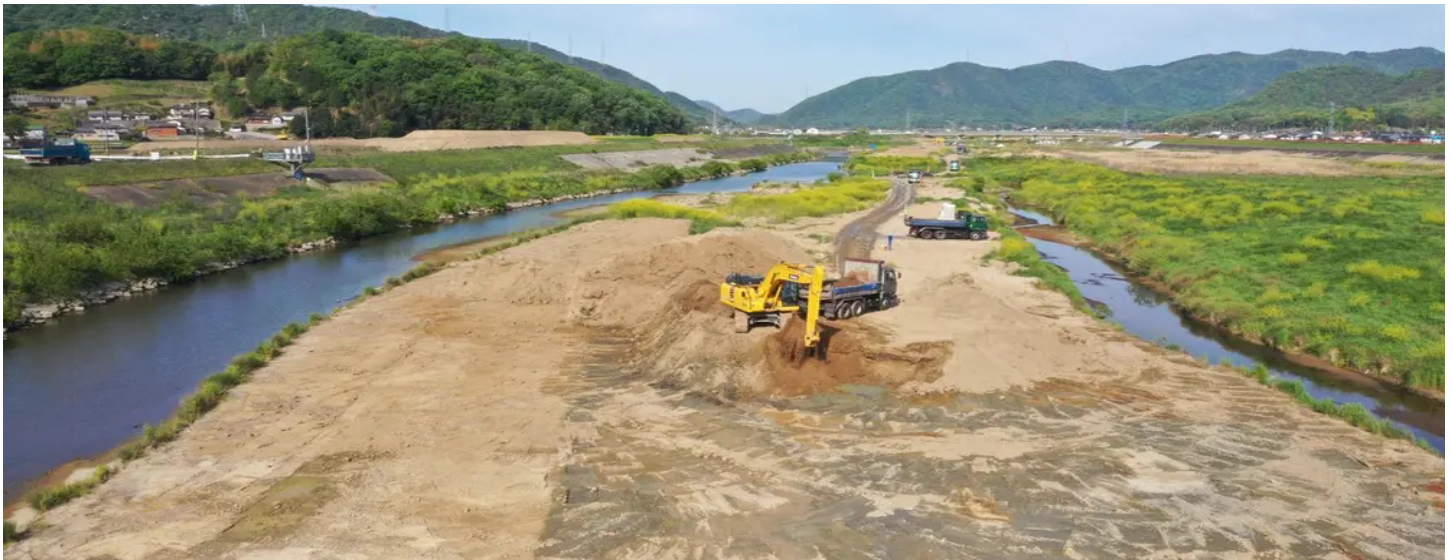
PICTURE 2: Excavation of the river channel to increase flow capacity (source: MLIT Mabi Bureau)
